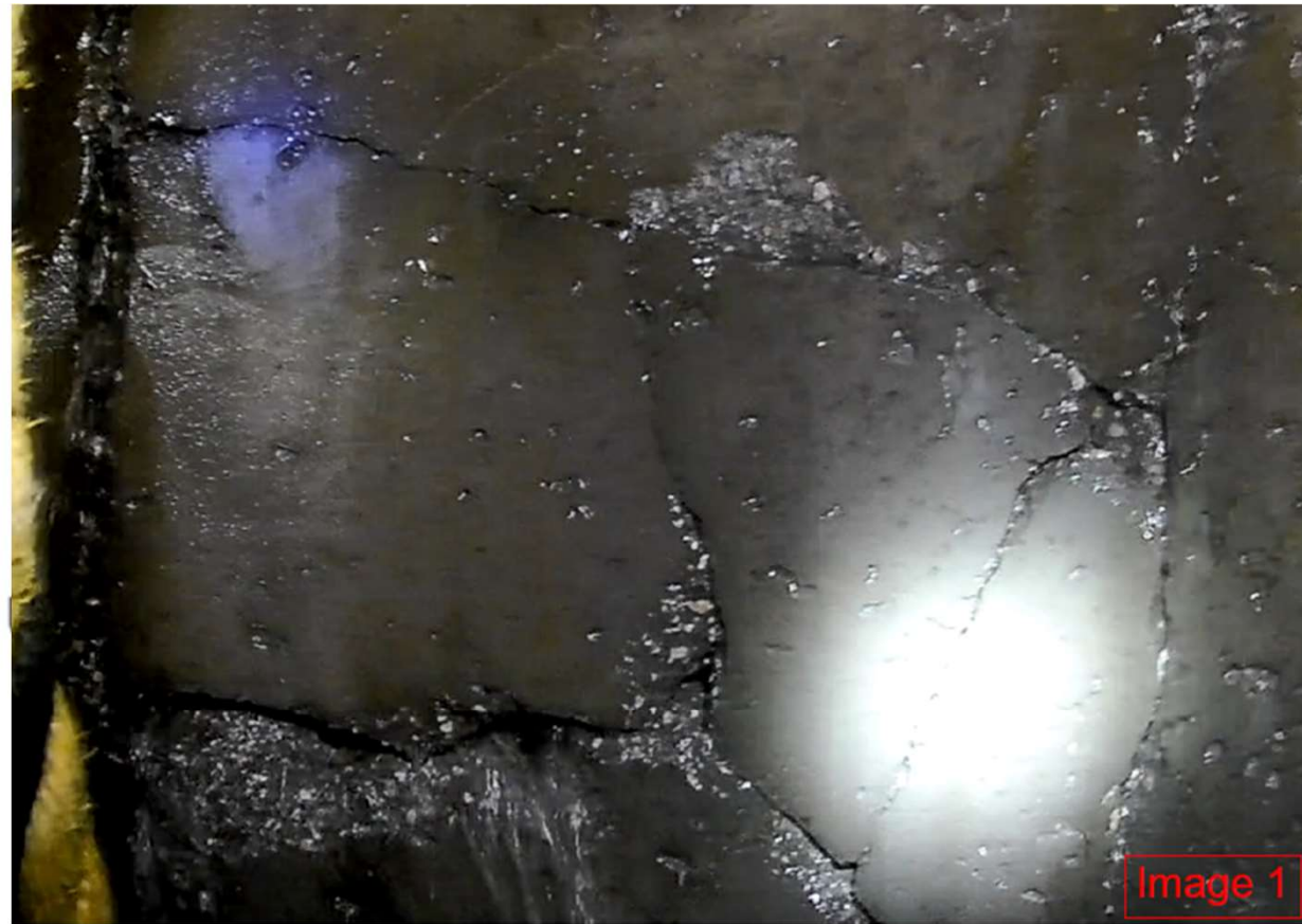
Image 1 taken at approximate elevation -14ft. Vertical and horizontal cracking with . Water intrusion is evident.
